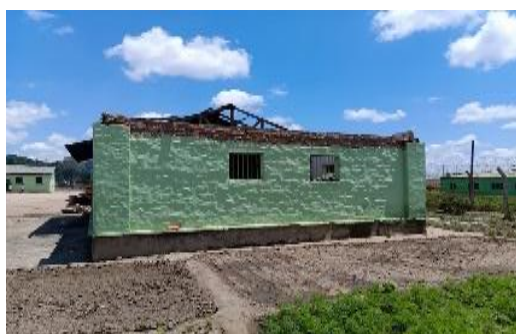
Blown off roof on the classroom block at Mukobeko Medium Facility
