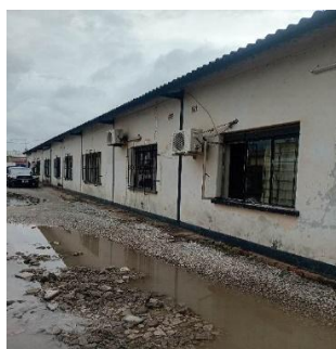
Wall not painted
