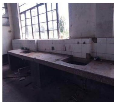
Dilapidated sink /Washing bench - Sinazongwe – Non - Functional Abattoir, Southern Province
