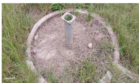
Non-functional borehole at Lucheche day secondary
