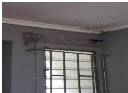
Stained wall and ceiling boards
