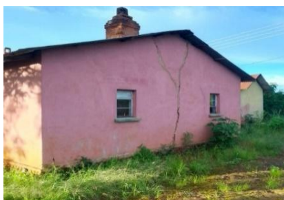
Lunzuwa FTC- cracked wall
