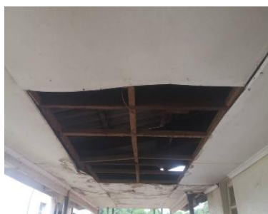
Broken ceiling – Kapata Urban Clinic Chipata
