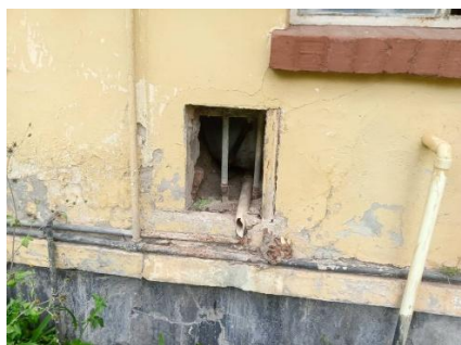
Worn-out plumbing system
