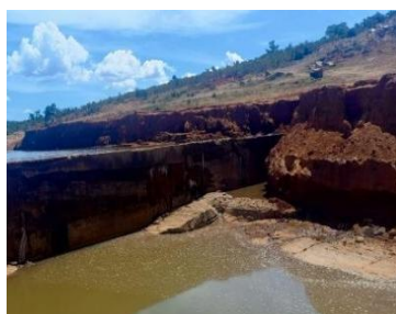
Washed Away Embankment Under Construction
