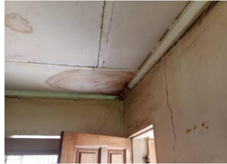
Stained ceiling board & cracked wall
