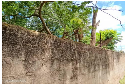
Damaged Electric Fence
