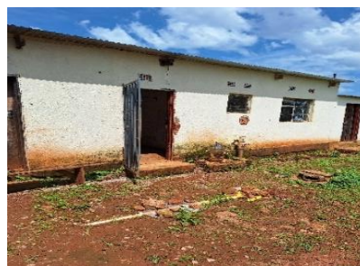
Solwezi Teachers College Clinic – Poorly Maintained
