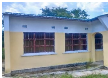
Windowpanes not fitted
