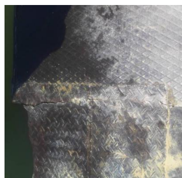
Damaged base - Lukulu Pontoon
