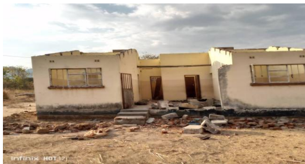
Camp House with a removed roof at Mbozi
