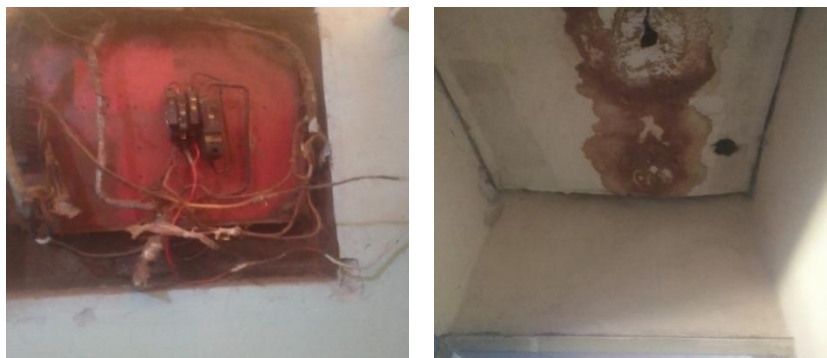
Naked wires and stained ceiling at Chipata Central Facility
