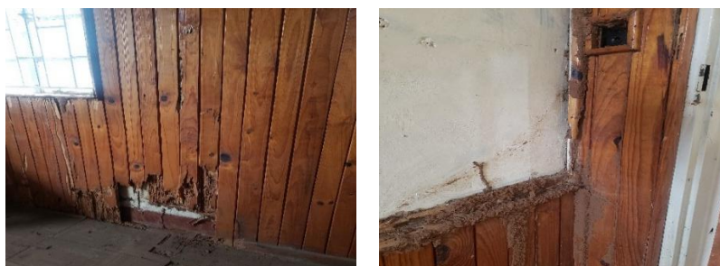
Termites on Wood Cladding
