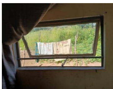
Fallen Burglar Bars
