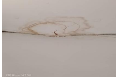
Damaged ceiling board
