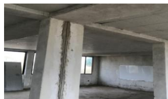
Cracked and Warped Bottom and Top Beams
