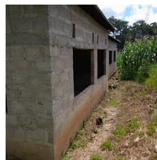
Stalled works - back view
