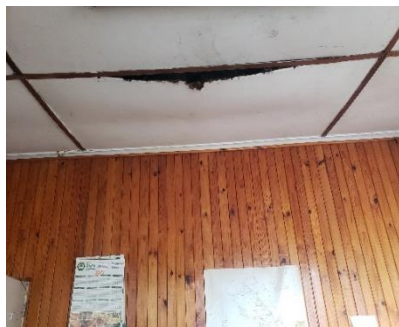
Falling Ceiling Board
