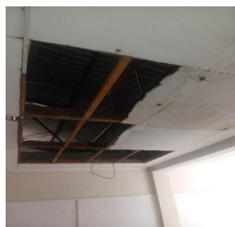
Broken ceiling board in the conference room
