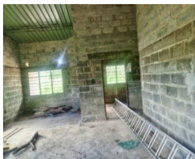
Interior walls not plastered
