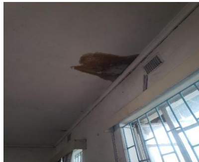
Damaged Ceiling Board due to leaking Roof
