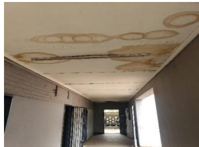
Stained ceiling board due to leakages
