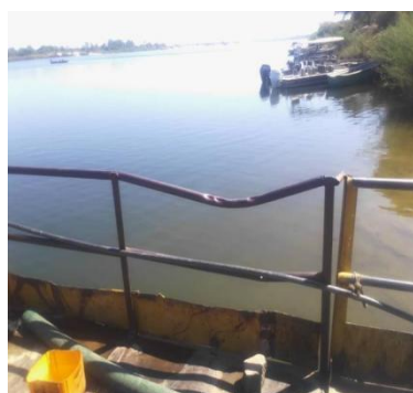
Damaged rails - Watopa Pontoon
