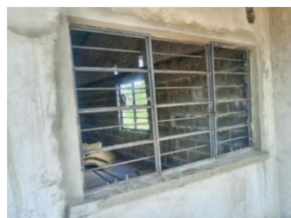
Windowpanes not fitted
