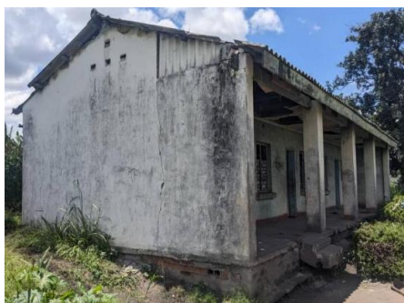
Dilapidated office block at Nsombo Veterinary Camp
