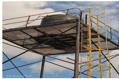
Non-functional water tank
