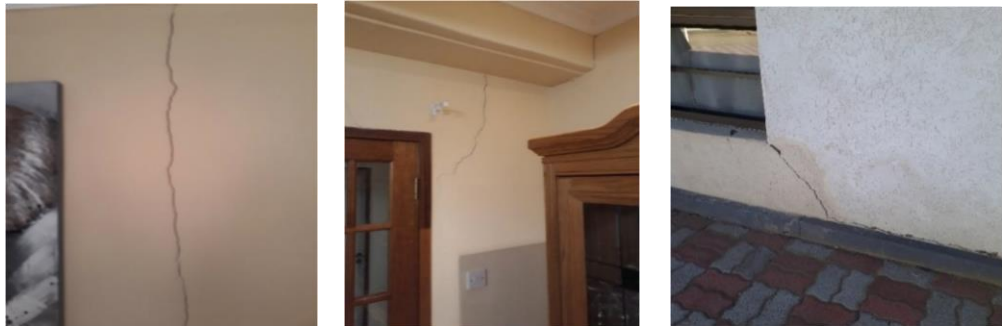
Cracks can be seen inside and outside the house
