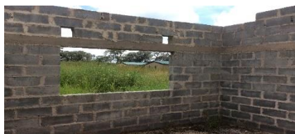
Incomplete camp house structure
