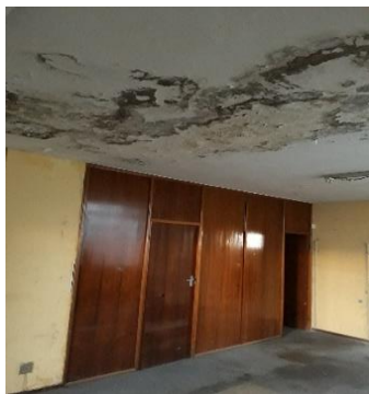
Ceiling falling off
