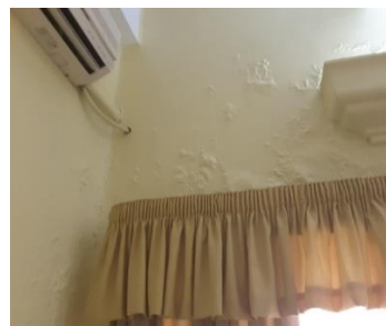
Leakages in the dining room
