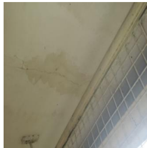
Crack on veranda wall
