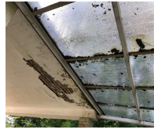
Falling ceiling board on the veranda
