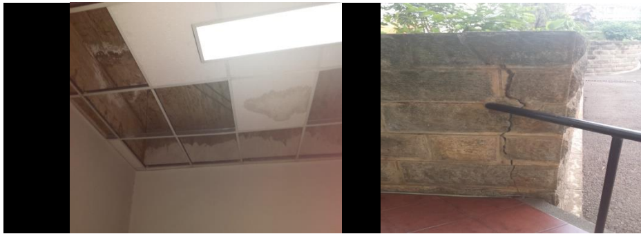
Leaking roof in one of the offices
