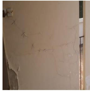
Cracks on balcony wall
