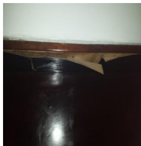
Peeling board in sitting room
