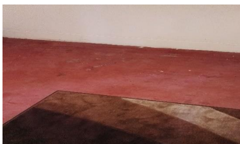
House No. 1 floor without tiles
