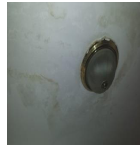
Leakages in the sitting room
