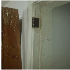
Damaged kitchen door
