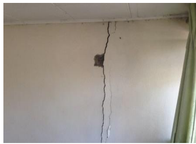
Cracks on the wall along the corridors
