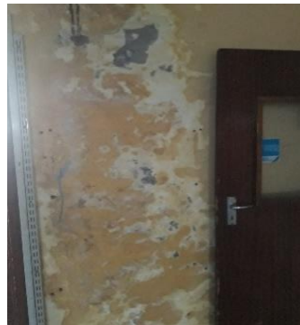
Paint peeling off
