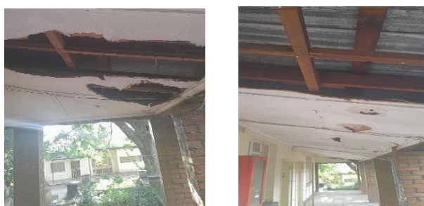
Dilapidated Ceiling Board
