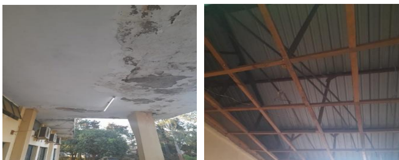
Dilapidated ceiling and leaking roof
