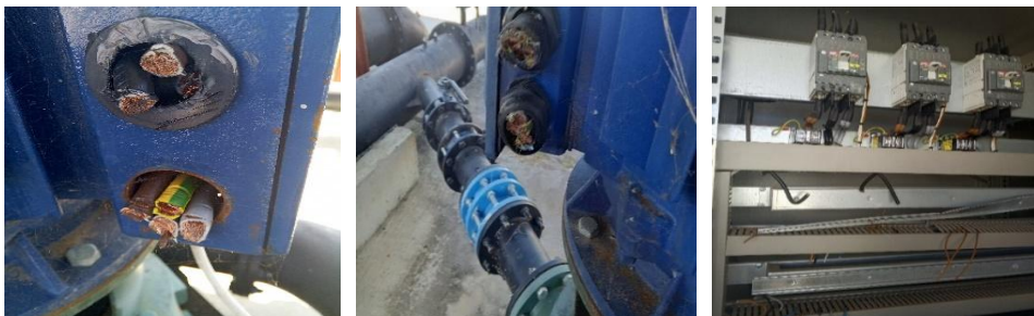
Vandalized copper cables and jumper cables from the pump station motors to the control panel
