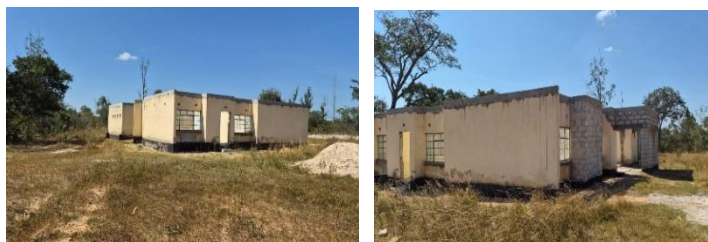
Abandoned works – office block
